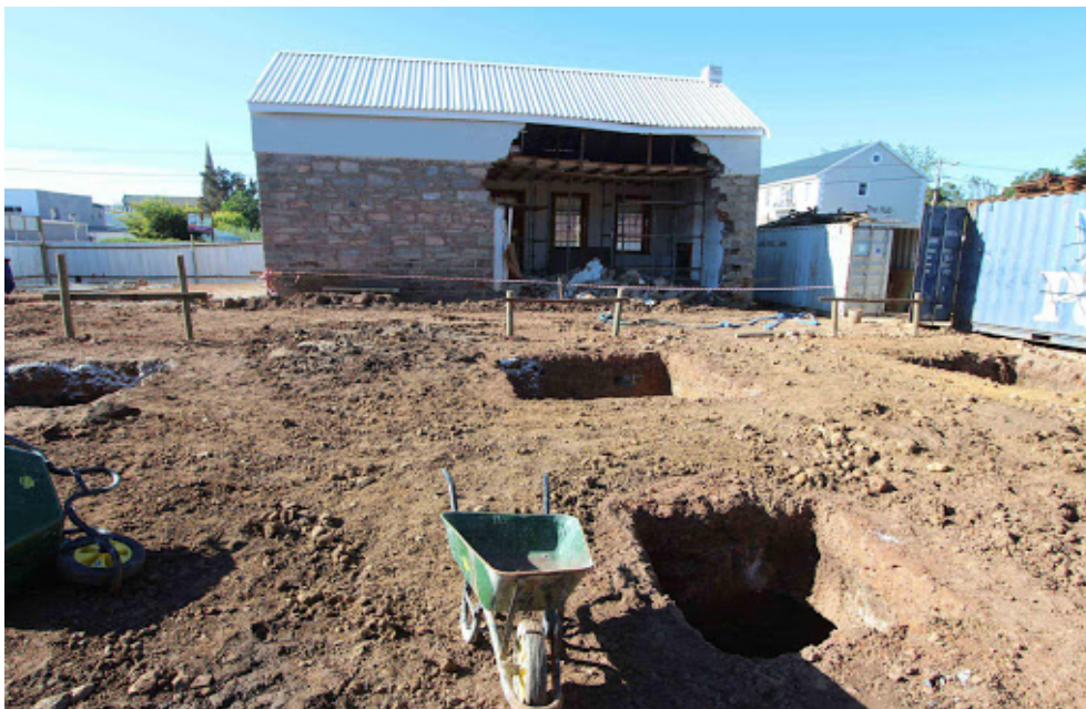
Figure 6. SuperSPAR construction illustrating damage to the historic property in Rose Street
