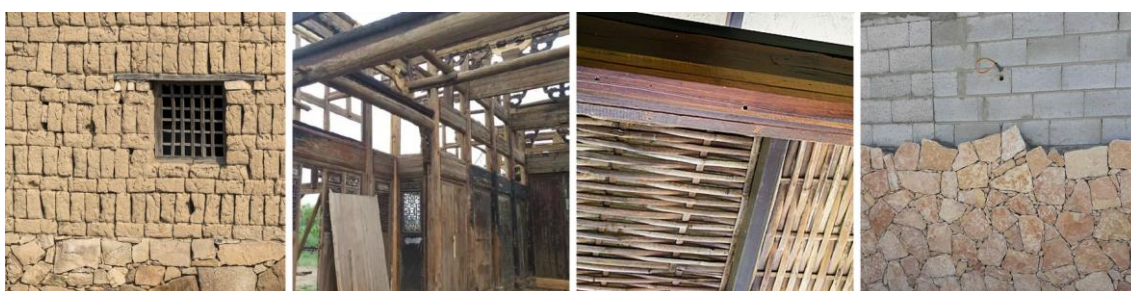
Fig. 104 Rammed Earth Wall, Wooden Structure, Bamboo Material and Stone (Drawn by the author)
