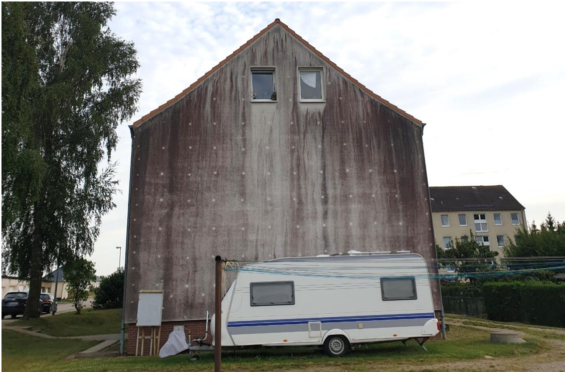
Figure 2: North gable near Wismar/Germany with pronounced infestation (Photo: author)
