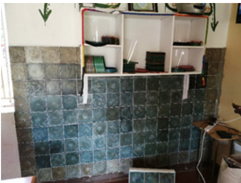
▲ Picture 5. Wall tiles representing 650 recycled soda and water plastic bottles at TakaTaka Plastics office in Gulu, 21st May 2021, author's photo
