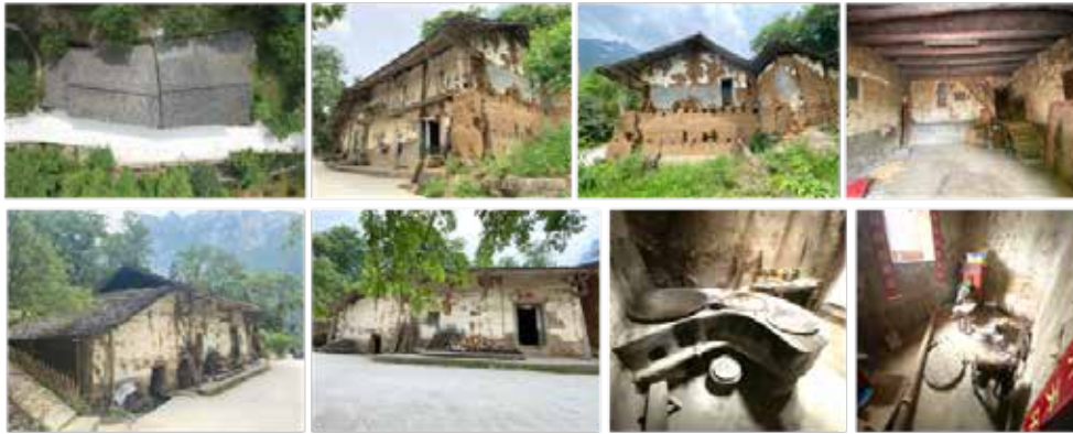
Buildings 2+3: The main body of the buildings are basically reserved and inhabited. It is recommended to repair and consolidate the building structure
