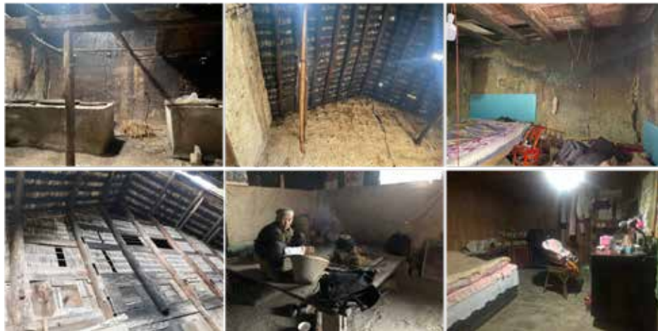
Fig 4.39: Disadvantages of the interior space of the building (source: photo by author)
