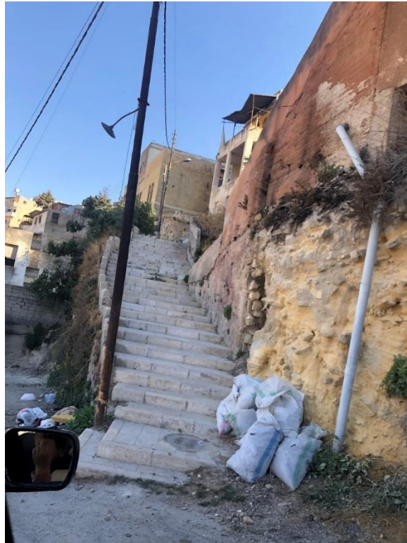
Figure 5.33: Dangerous stairs in Salt city
