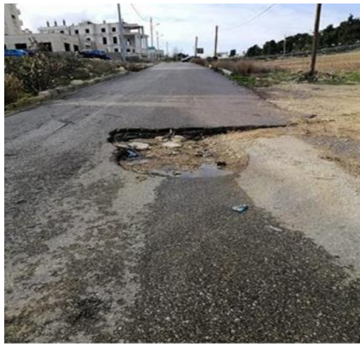
Figure 5.35: Unmaintained Street in Salt city cause dangerous accident
