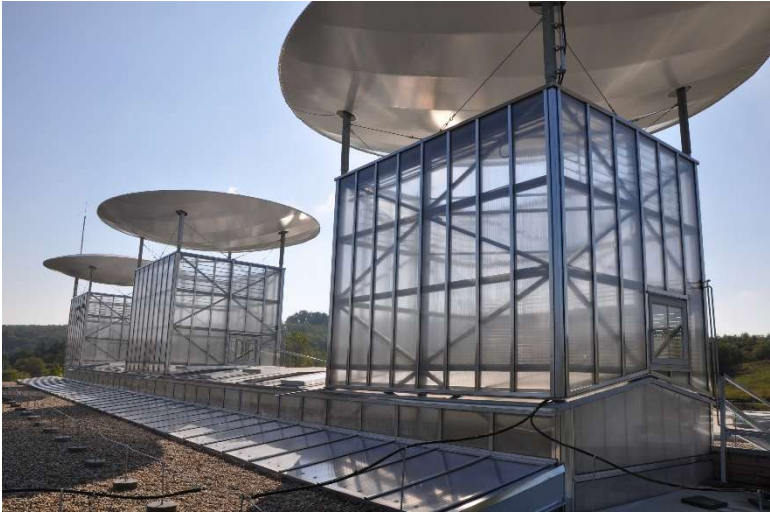
Figure 54. Practical application of Venturi plates at the production hall of RATI Ltd. in Komló
