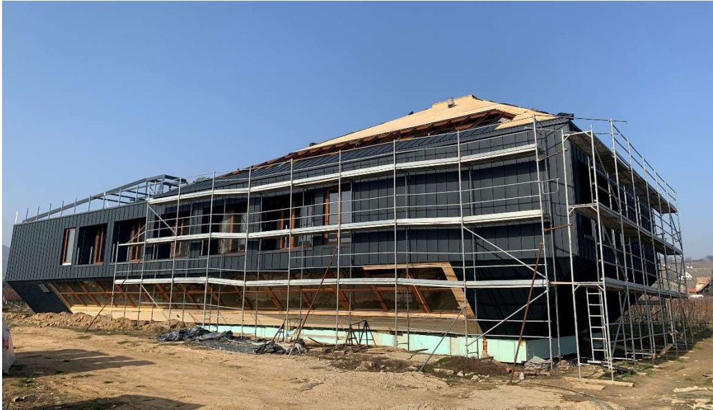
Figure 46. The prototype building under construction with the wind_catcher inlet (left pyramid) and the ‘Venturi’ outlet structures (right pyramid)
