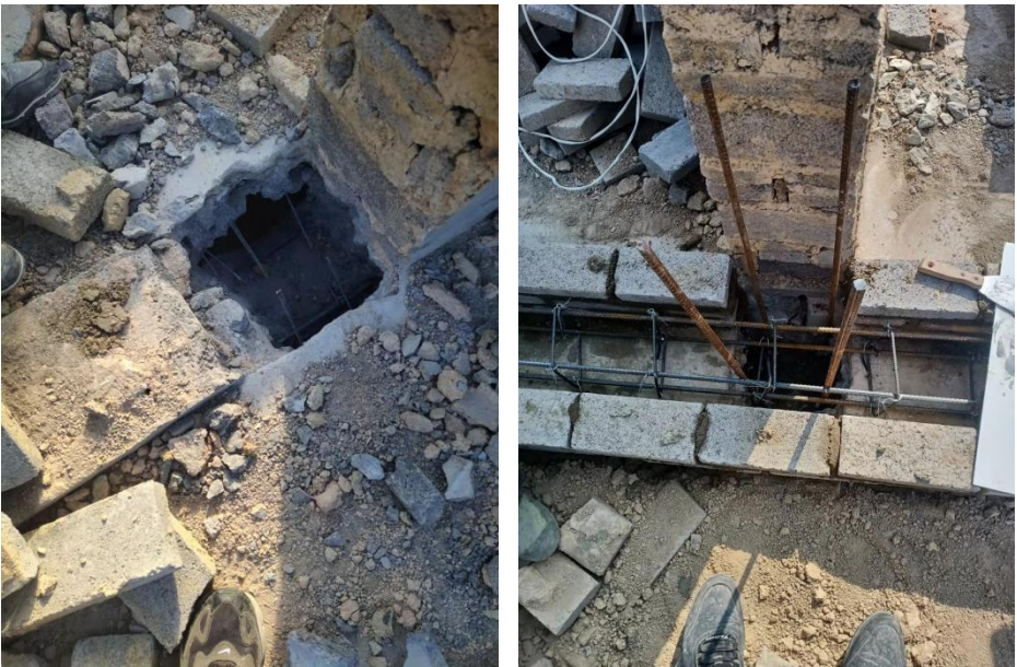
Column structure reinforcement on the second floor (Source: photographed by the author)
