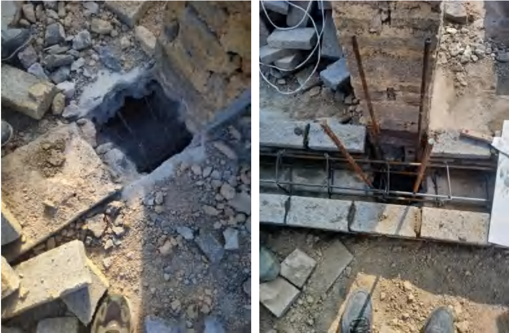
Figure 5-26. Column structure reinforcement on the second floor (Source: photographed by the author)
